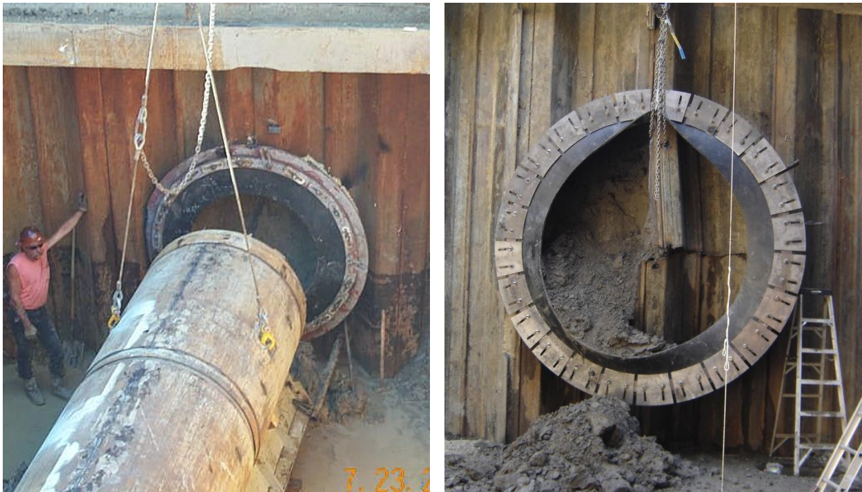
Figure 14. Left: MTBM Launch through Entry Portal. Right: Shoring Removal from Exit Portal in Sheetpile Shaft with Gasketed Seal.
