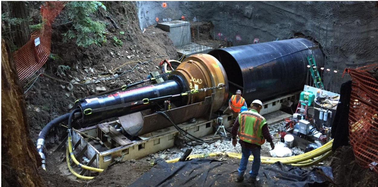
Figure 10. Lubrication Pipe Attached Near Top of Pipe. Adaptor Cone to Transmit Hammer Forces to Casing
